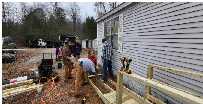
Sylva United Methodist Church, Building a ramp for the elderly, Courtesy of Department on Aging
